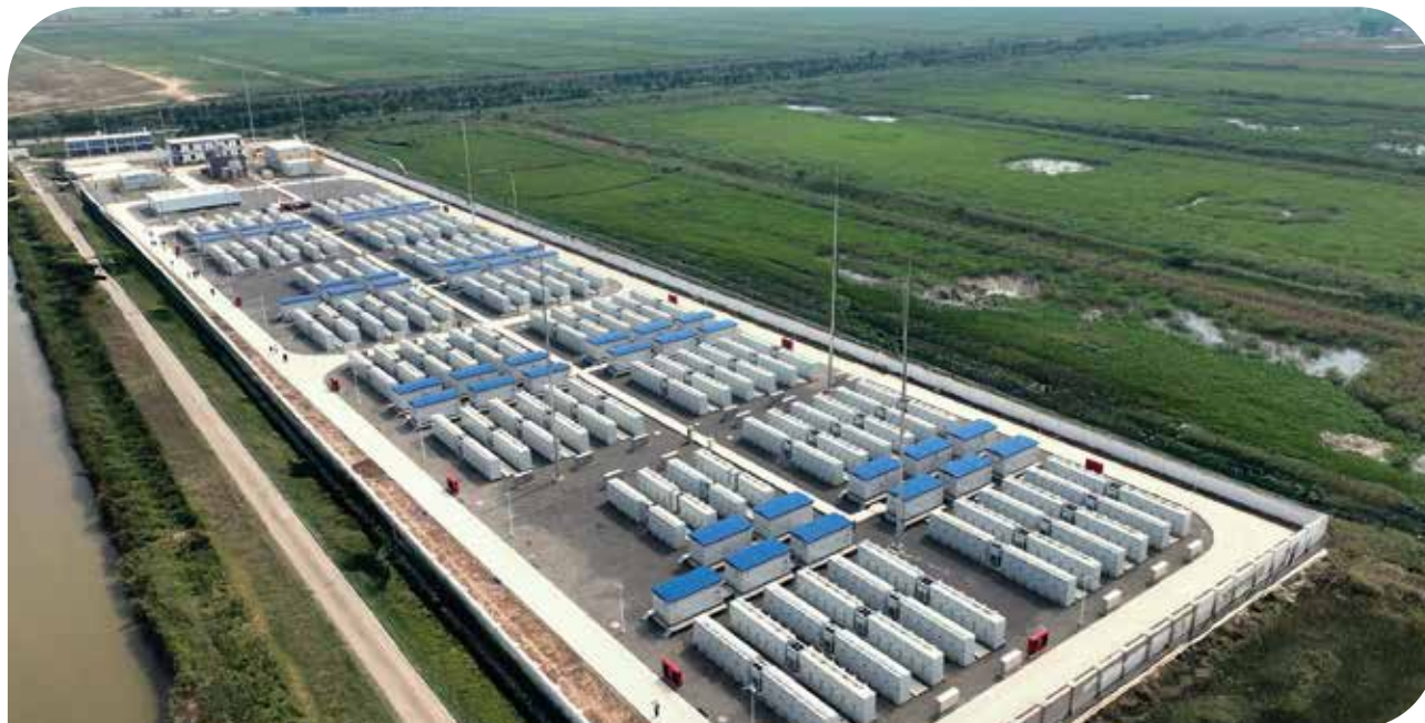
2 Model: ORION UE-L400 Capacity: 200 MW/400 MWh Binhai, Tianjin, China
