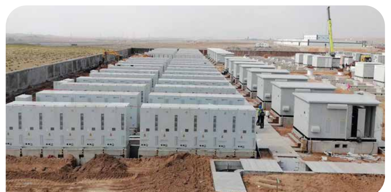
4 Model: ORION UE-L400 Capacity: 50 MW/100 MWh Ningxia, China
