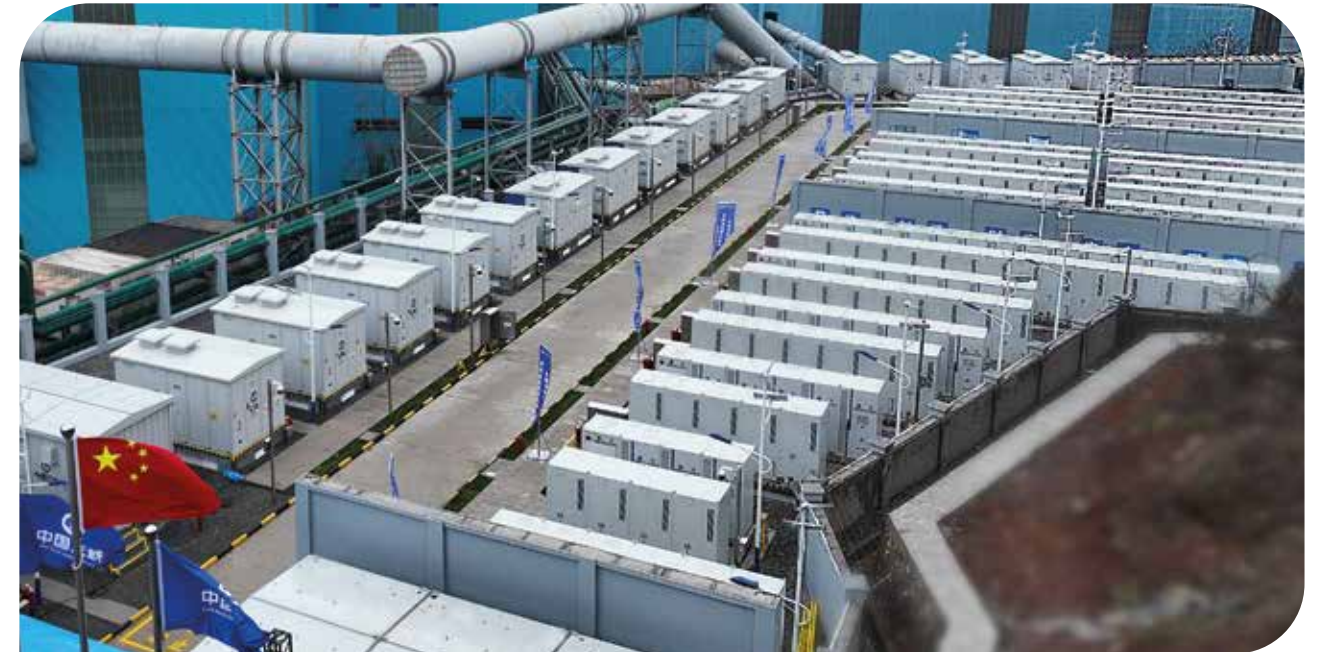
3 Model: ORION UE-L400 Capacity: 61 MW/123 MWh Nanjing, Jiangsu, China
